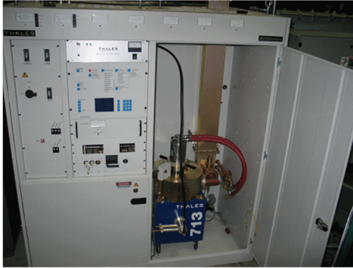
Figure 4.4.3: IOT inside the transmitter.
