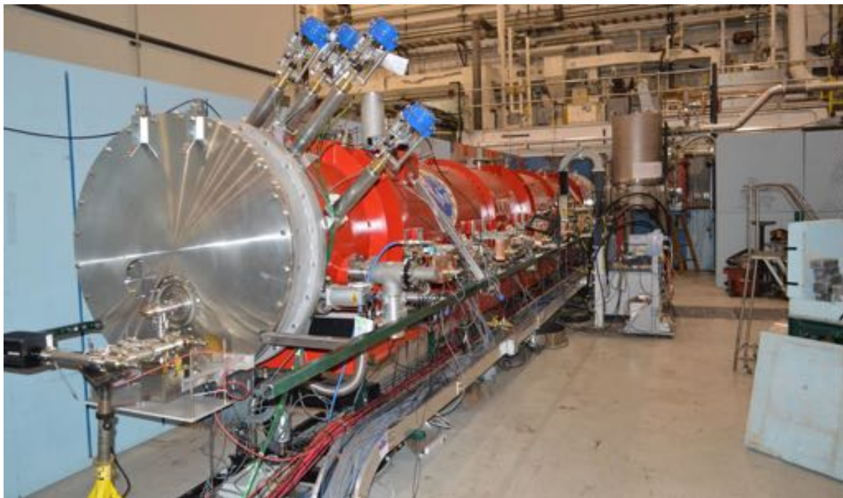
Figure 1.3.3: The Cornell Main Linac Cryomodule (MLC) installed for RF testing in the experimental hall L0E.
