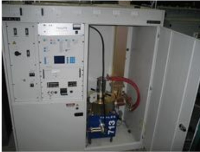
Figure 4.4.3: IOT inside the transmitter.
