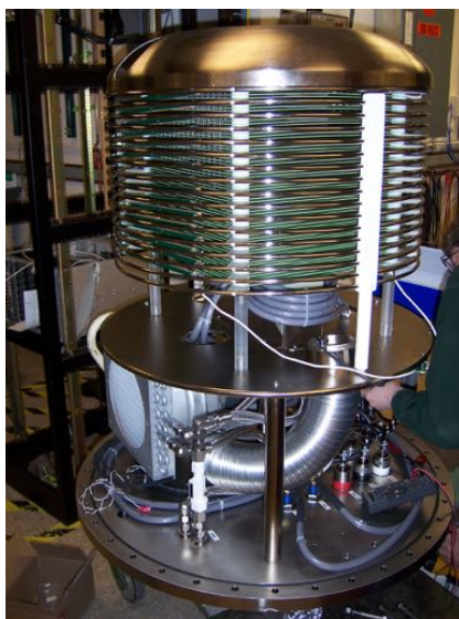
Figure 4.2.4: The HV section of the 750kV power supply. Individual circuit boards are visible inside the potential grading rings. The primary winding of the insulating core transformer is the large diameter gray-insulated wire below the circuit boards. The HV section is mounted in the pressurized SF 6 tank with its axis parallel to the axis of the gun ceramic.
