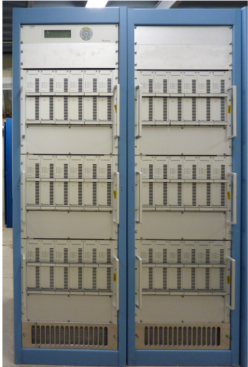
Figure 2. Danfysik Power Supplies
