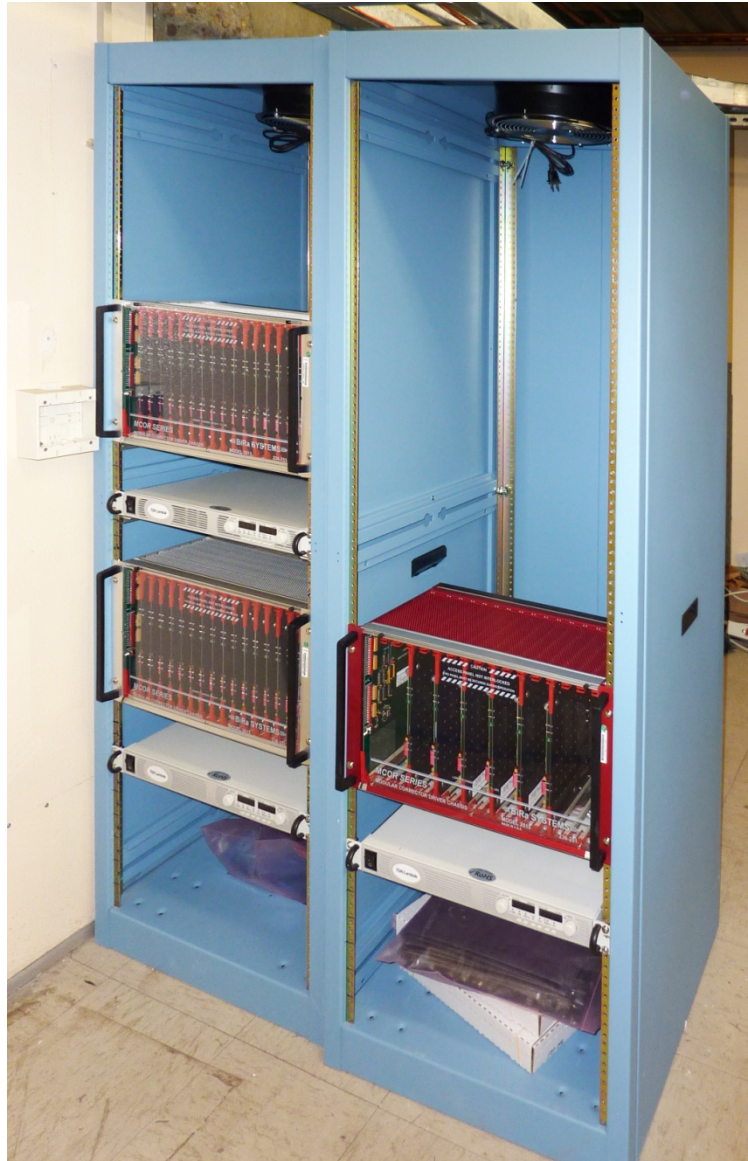
Figure 3. BiRa Power Supplies
