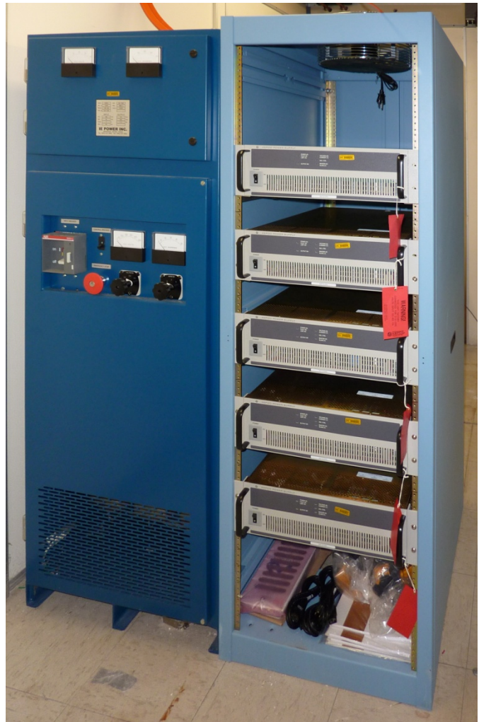
Figure 1. IE Power & Kepco Supplies
