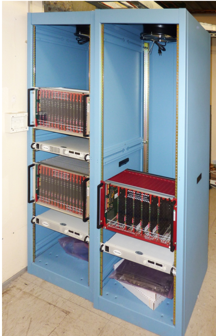
Figure 3. BiRa Power Supplies
