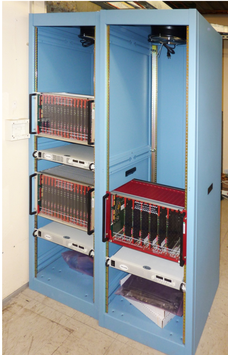
Figure 3. BiRa Power Supplies
