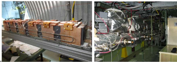
Figure 1: Abort Kicker Magnets System in RHIC
