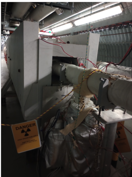
FIG. 2. Upstream side of the beam dump (5 January 2024).
