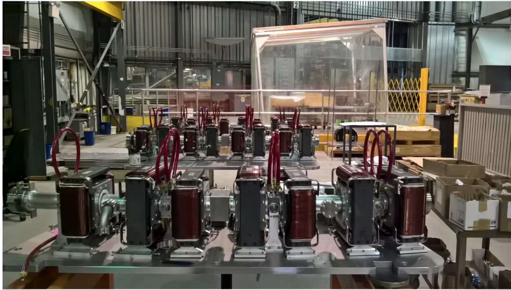
Figure 0.9.13: The FFA magnets are installed on the girders after the field correction is finalized.
