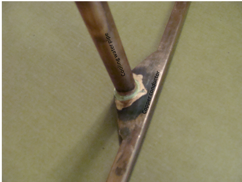
Figure 22: A picture of the brazing connection of one of the cooling pipes with one of the four conductors of the coil.
